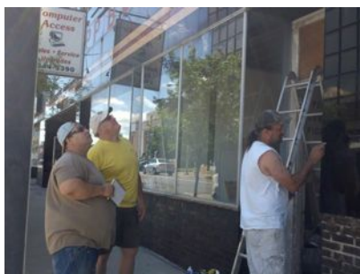
L-R: Hank Falkenberg, vitrolite apprentice and owner Kent Renshaw check out the vitrolite above the storefront windows. Harry Clark works on the new Vitrolite
